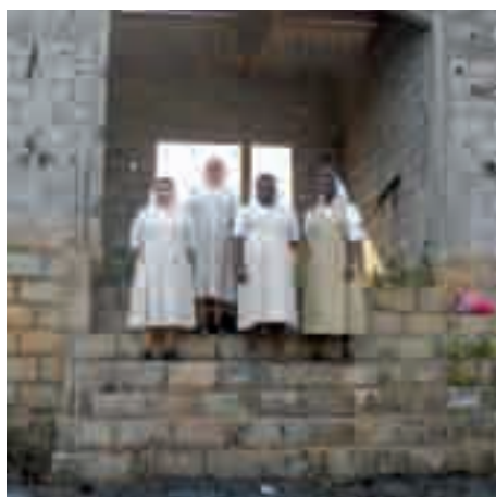
The bare walls have been built, but these Carmelites cannot live here yet.
